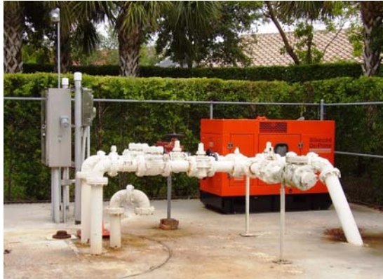
Emergency Bypass Pump
