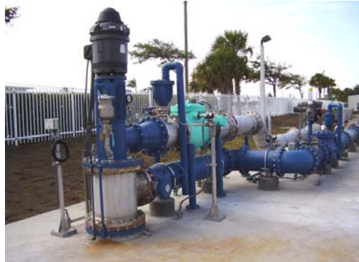
Aquifer Storage and Recovery well # 2
